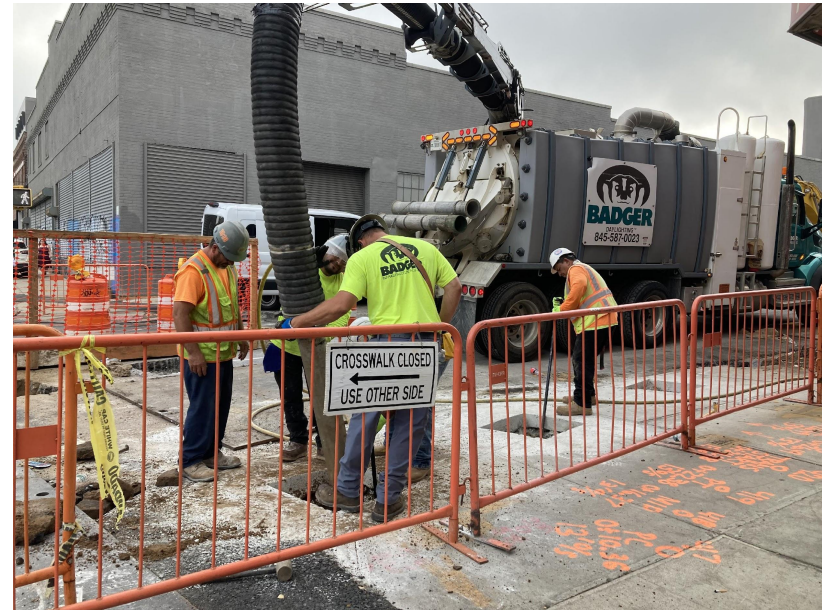
Sewer improvements in progress on 7th Street between 3rd and 4th Avenue September 2023
